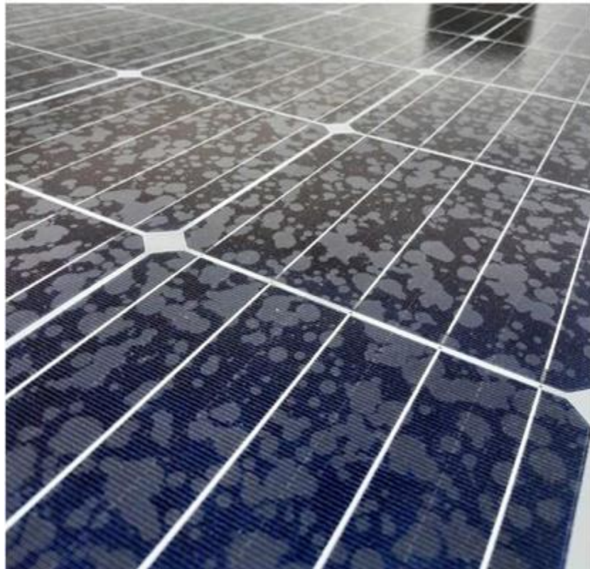
Fig.2 Moisture under the glass
