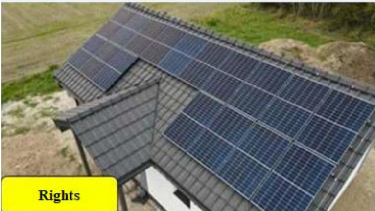
Fig.4 Example of photo documentation of a photovoltaic installation - REQUIRED BY THE MANUFACTURER
